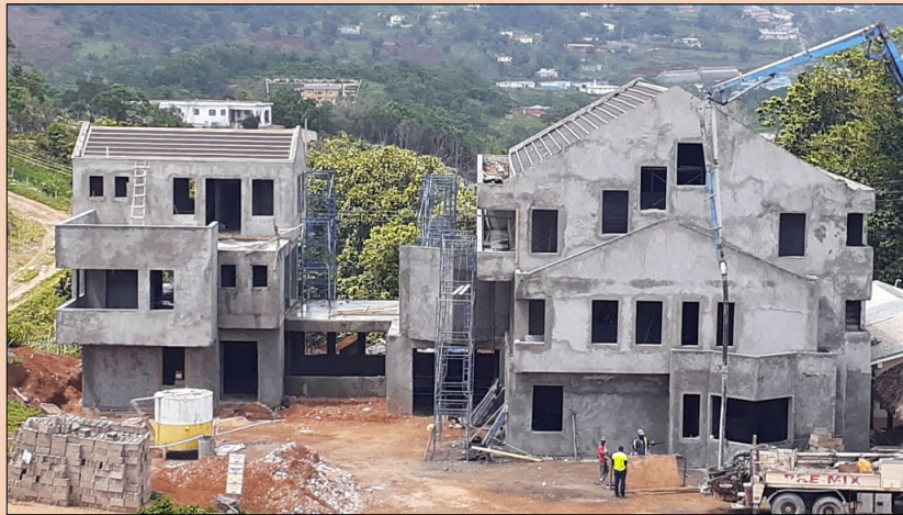
Good progress is being made on the new MOBH dormitory which will hopefully be completed by January 2021
